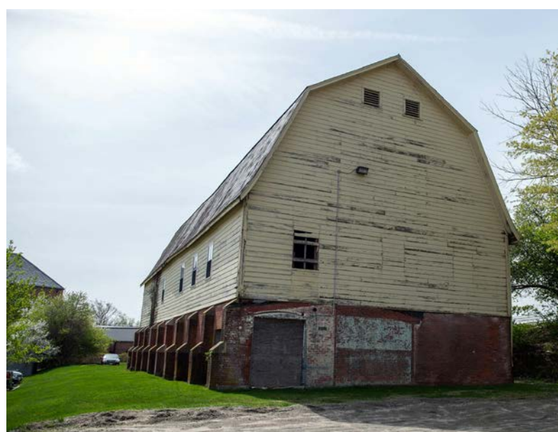
Signs of deterioration can be seen on UConn's yellow dairy barn.
